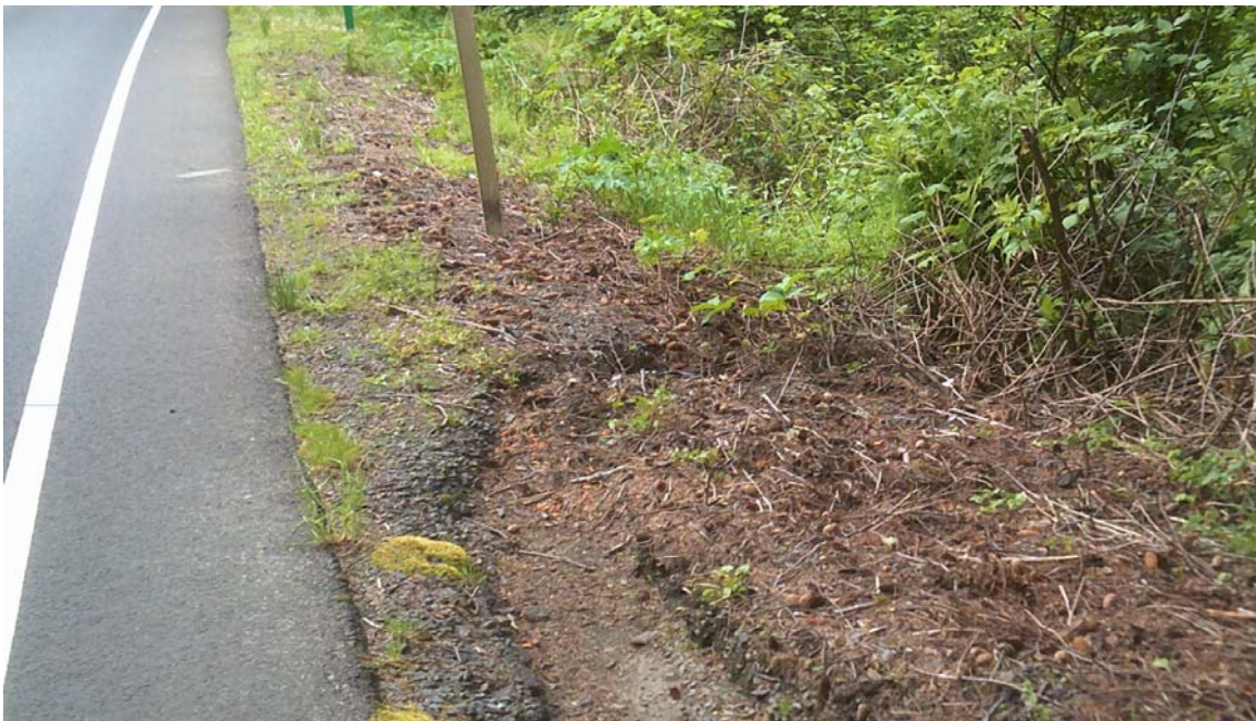
Figure 6 - Downstream end of existing open channel along roadside (Green stake in background marks location of culvert end crossing highway)
