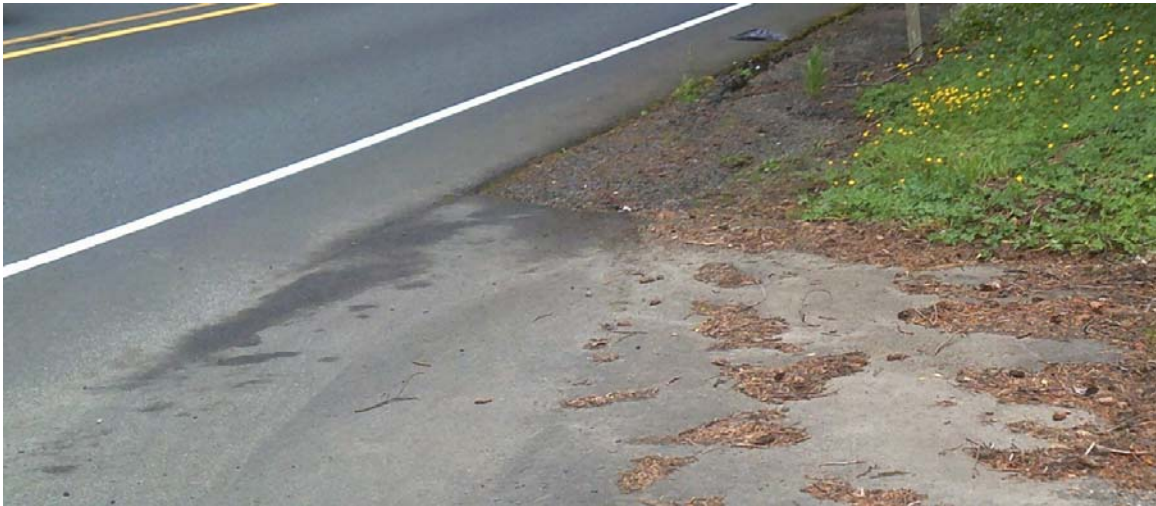
Figure 5 - Upstream end of existing open channel along roadside (Beginning of channel is visible approximately 6' from end of widened pavement)
