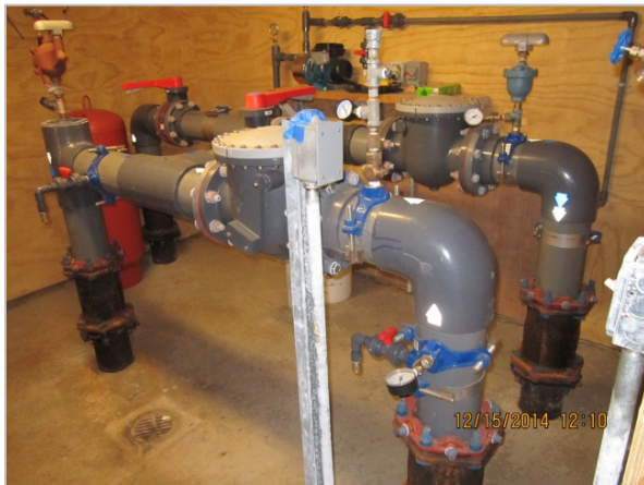
Photo 15: Flow Routing Assembly
