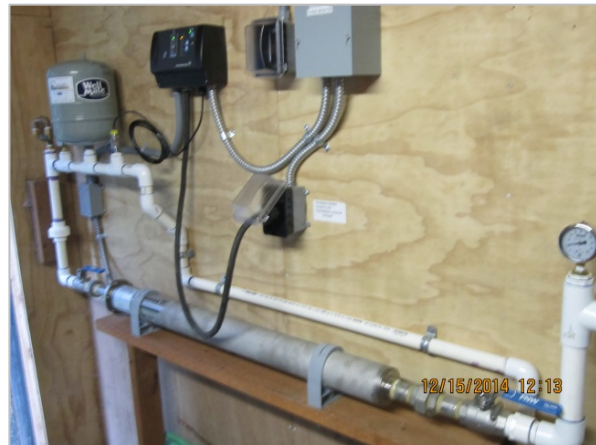
Photo 16: Pump (to "Mountain Zone")
