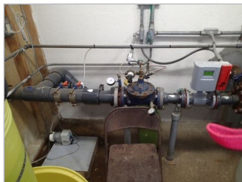
Photo 6: Flow Control Valve
