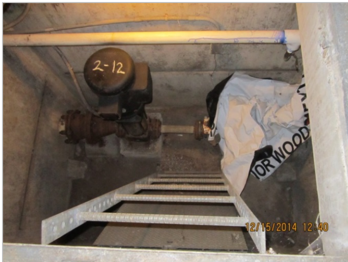
Photo 11: Pump Station (interior)
