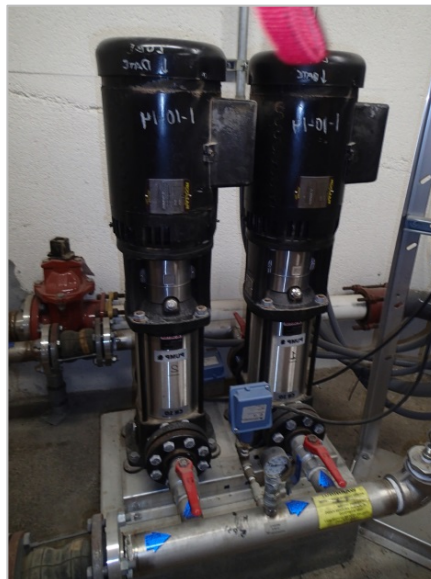
Photo 4: Pumps (to Upper Zone)
